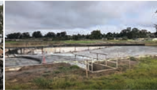
Aftermath — Remaining foundation
